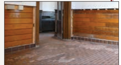
THE RECENT REMOVAL OF NON-HISTORIC 1980'S PANELING IN THE WAITING ROOM AREA REVEAL THE STATION'S ORIGINAL HORIZONTAL PLANK WAINSCOTING, STILL INTACT UNDERNEATH.
